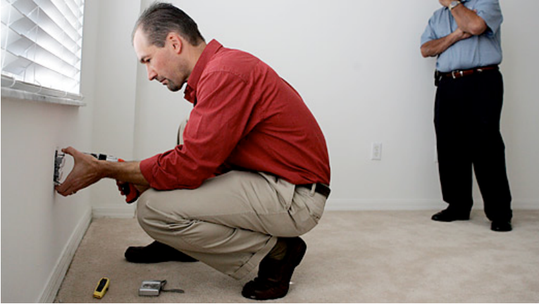
Howard Ehram of Chinese Drywall Screening removes an electrical plate to see if the receptacles show any signs of Chinese drywall in a home in Port St. Lucie, Fla.
